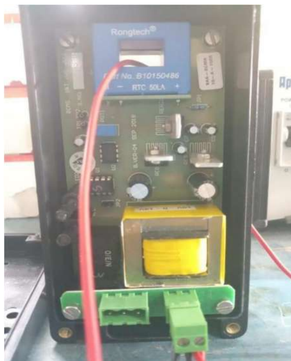
Fig. Battery Charging Monitoring System
