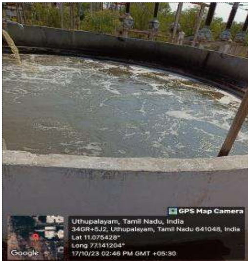
Sewage Treatment Plant
