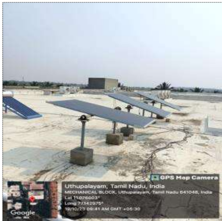
Solar Power System
